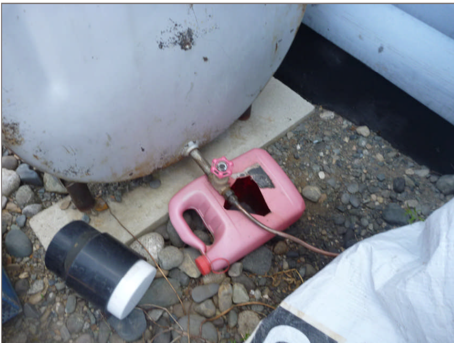
Photo 2: Hydrocarbon staining and leak collection at AST located at House 10
