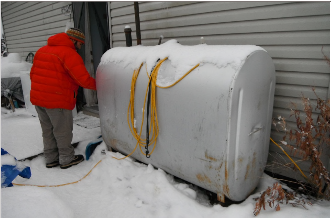
Photo 2: Typical Above Ground Storage Tank
