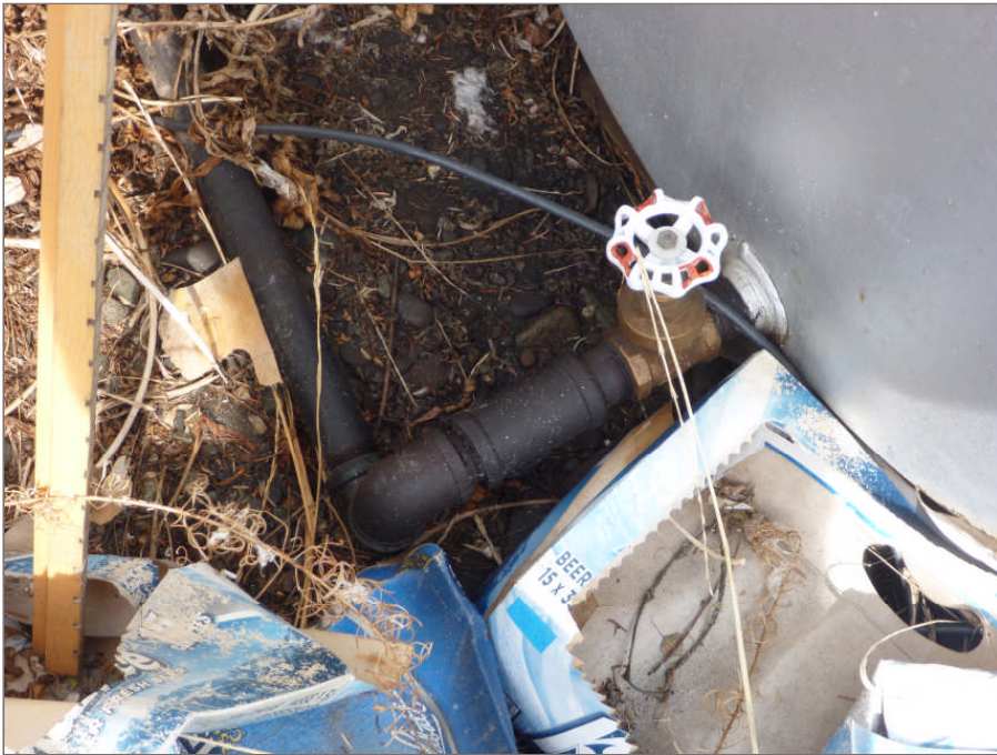
Photo 5: Hydrocarbon staining around southern most AST located at Duplex 16/17
