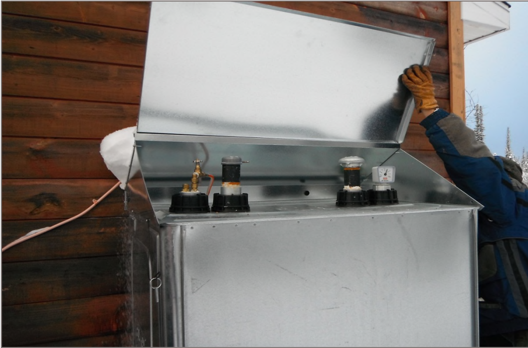
Photo 1: Double Walled Above Ground Storage Tank at House 5
