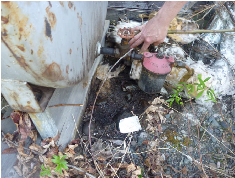
Photo 3: Hydrocarbon staining around AST located at House 12
