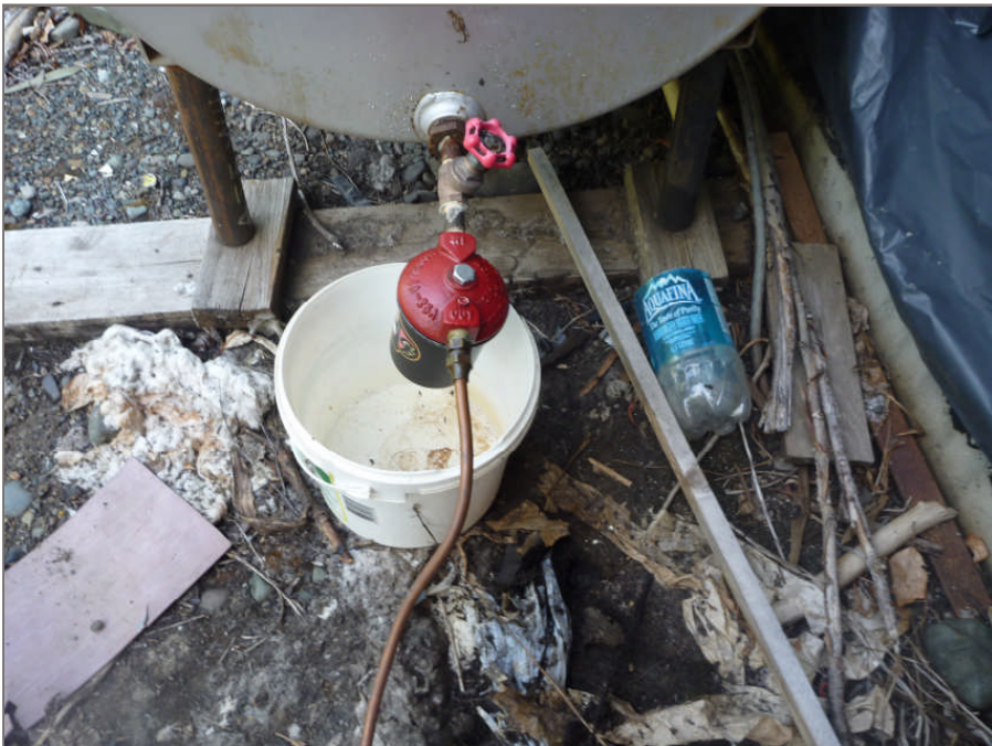
Photo 4: Hydrocarbon staining around AST located at House 13
