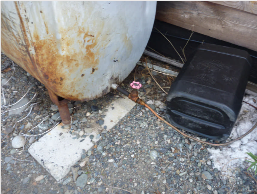
Photo 1: Hydrocarbon staining around AST located at House 4
